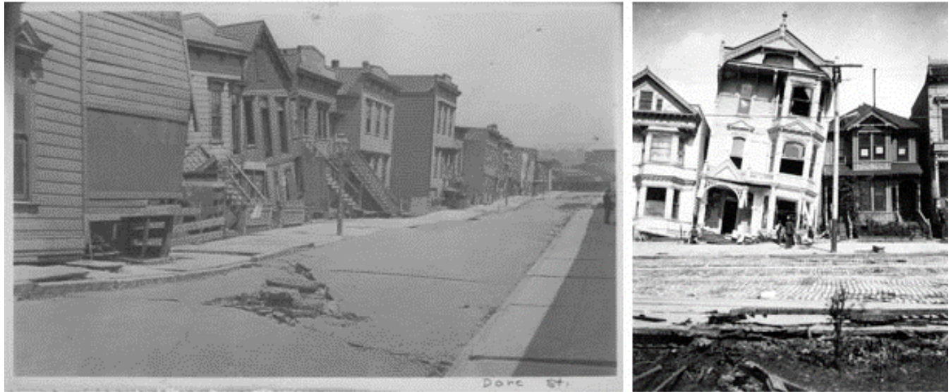
Figure 14.79 Photos Above Show Two Low Lying Areas in San Francisco After the 1906 Earthquake, Much Damage Was Contributed to Liquefaction. Image is in the public domain.
